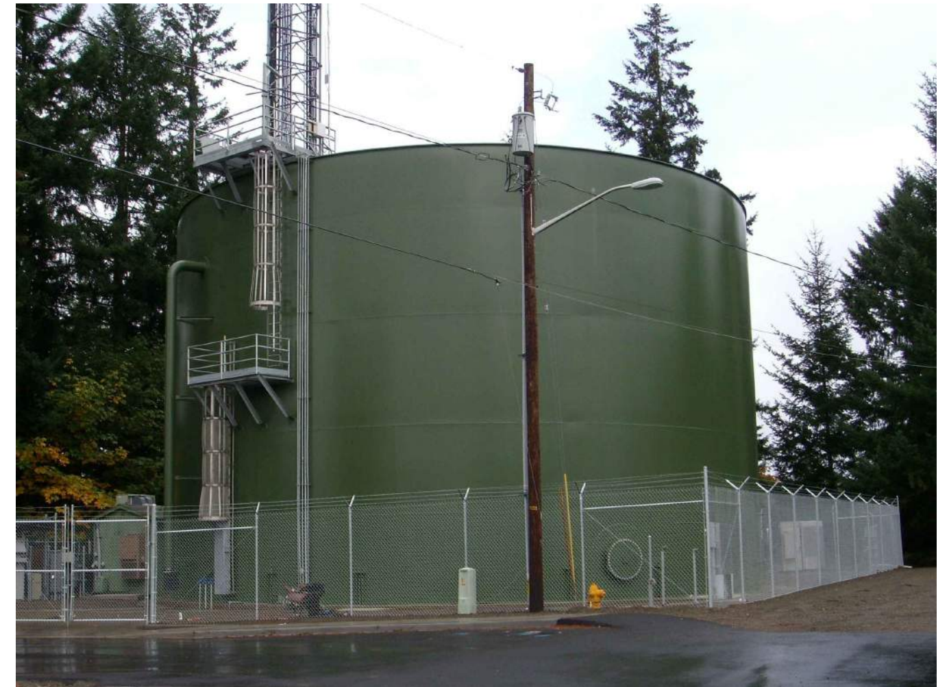
WELDED STEEL RESERVOIR PHOTO SOURCE: GRAY & OSBORNE
