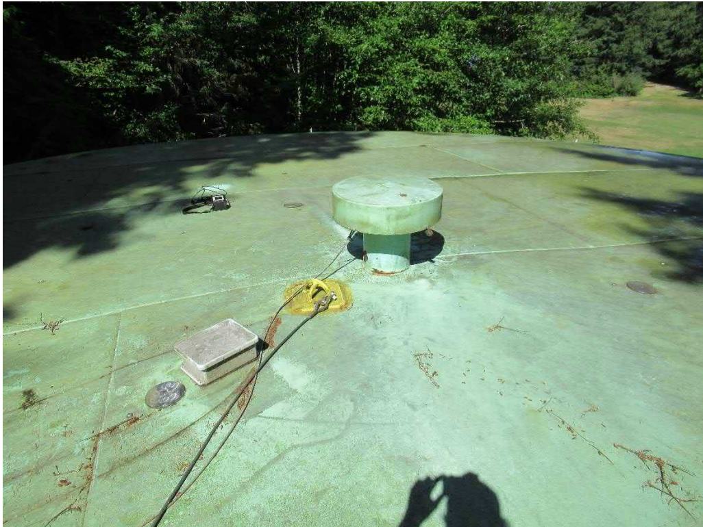
Photo 18: Anchorage, roof vent, and cathodic protection box.
