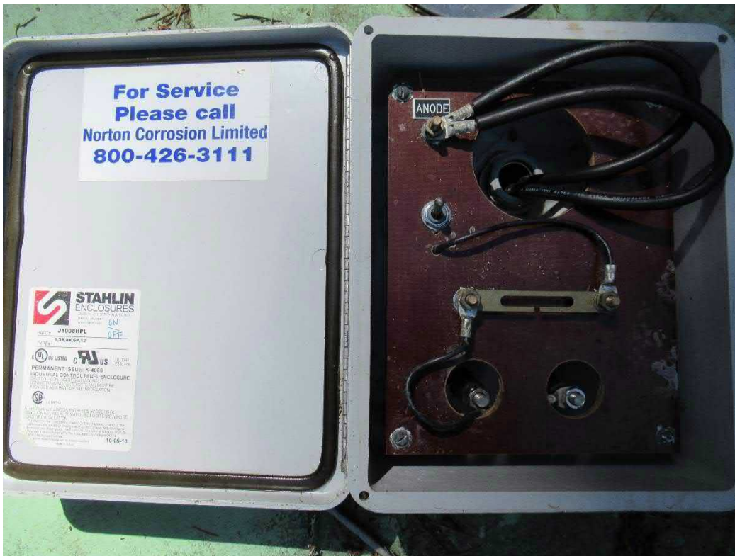
Photo 20: Cathodic protection box.
