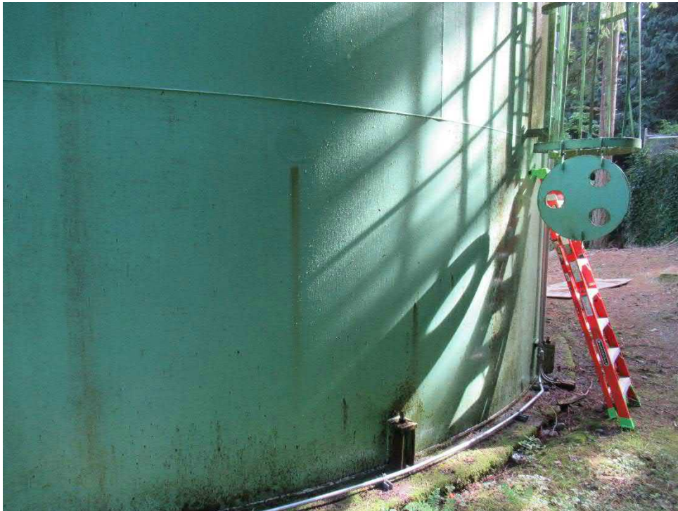
Photo 4: South side of tank with vertical swinging ladder guard.
