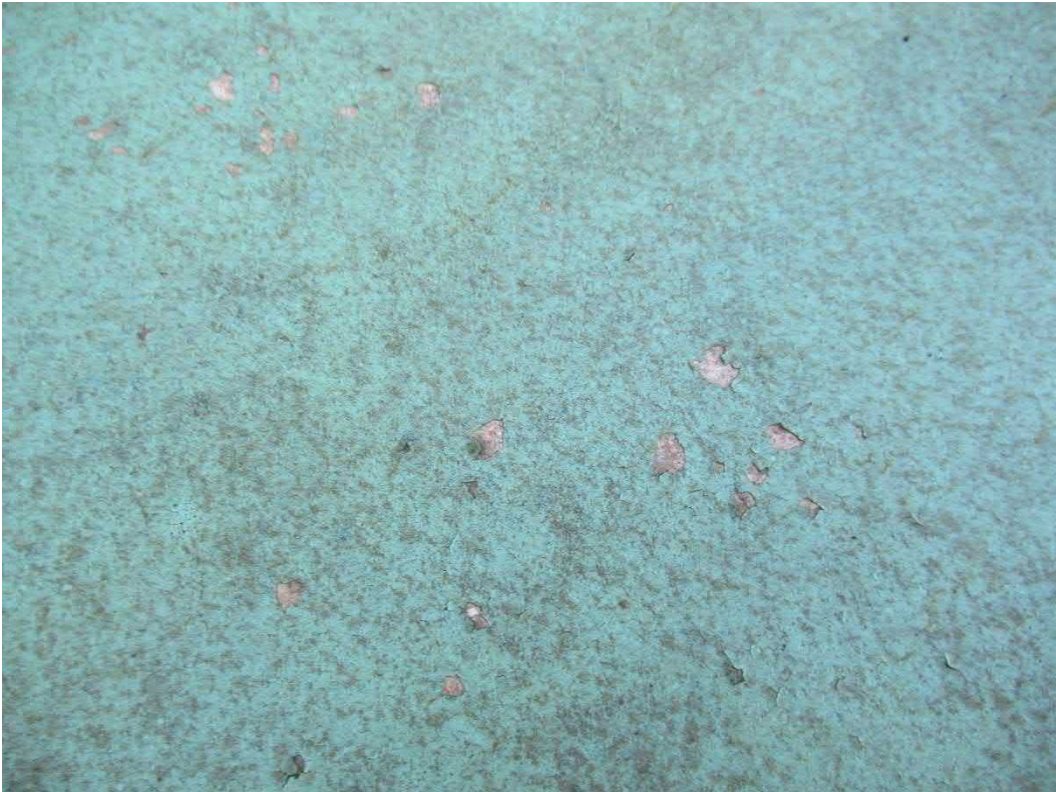
Photo 28: Coating delamination on the roof.
