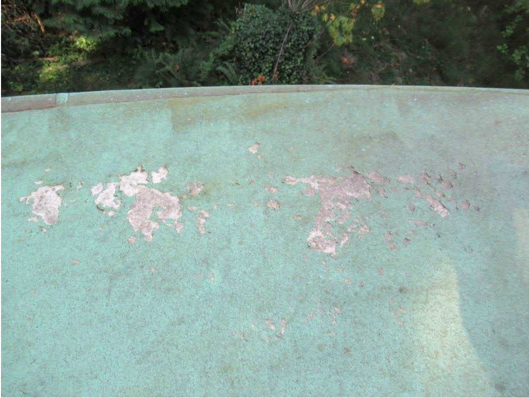
Photo 27: Coating delamination on the roof.
