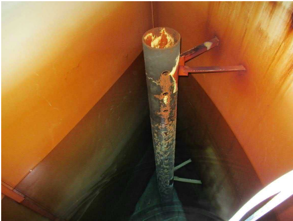
Photo 30: Inlet pipe diffuser.
