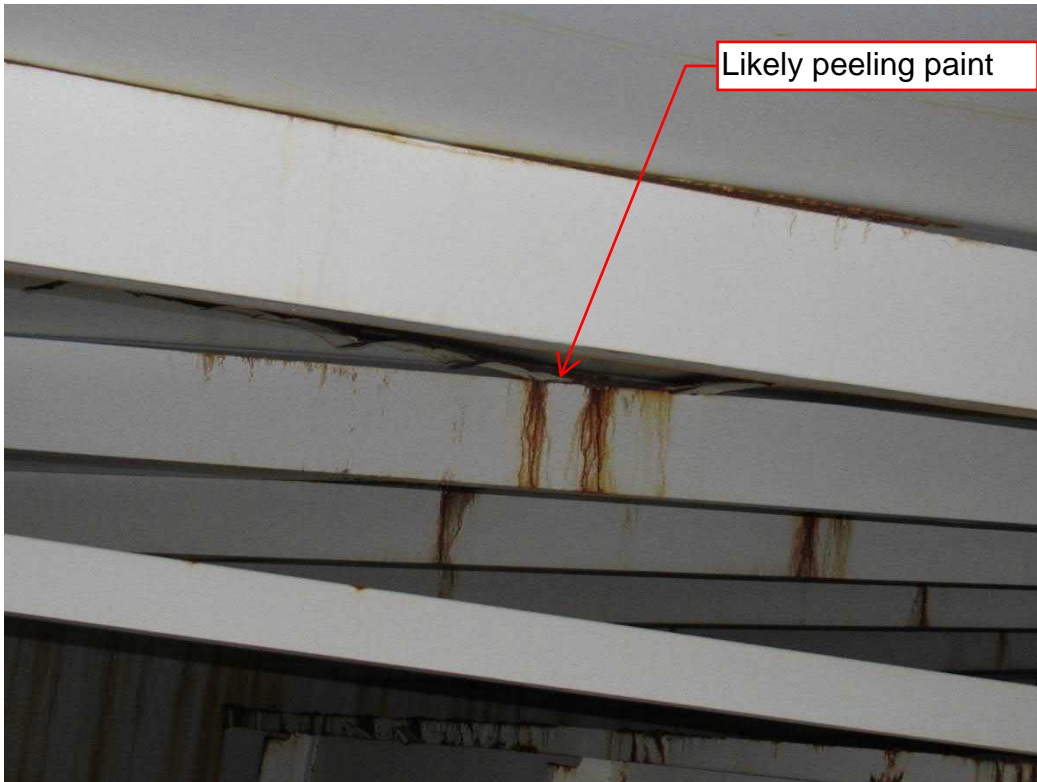
Photo 35: Interior condition. Note delamination in roof.
