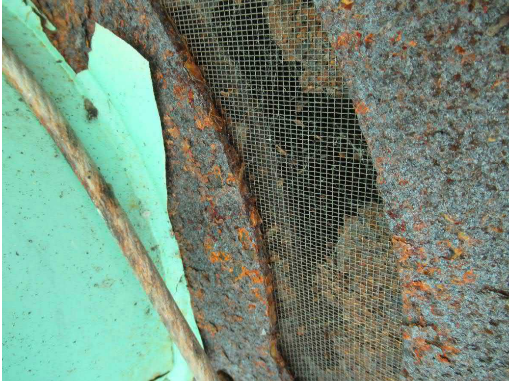
Photo 19: Roof vent with rust on the interior of screen.
