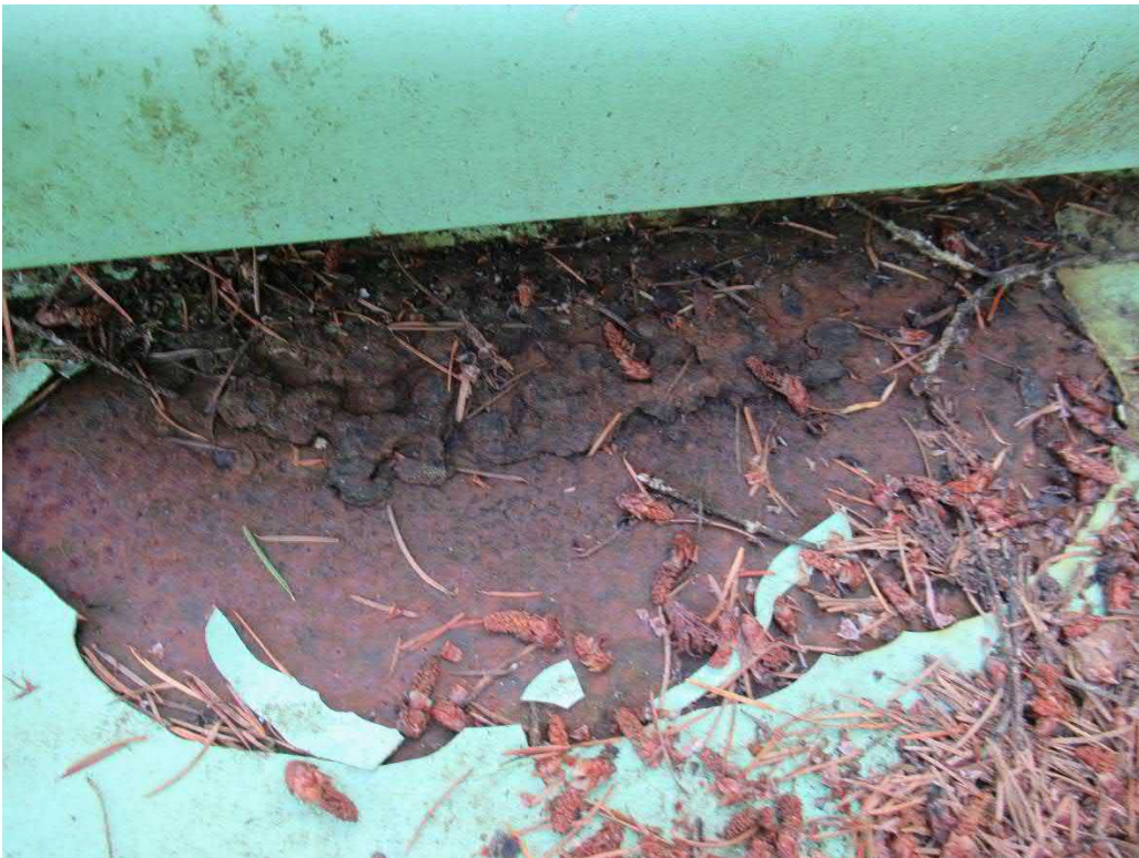
Photo 24: Corrosion adjacent to the access hatch.
