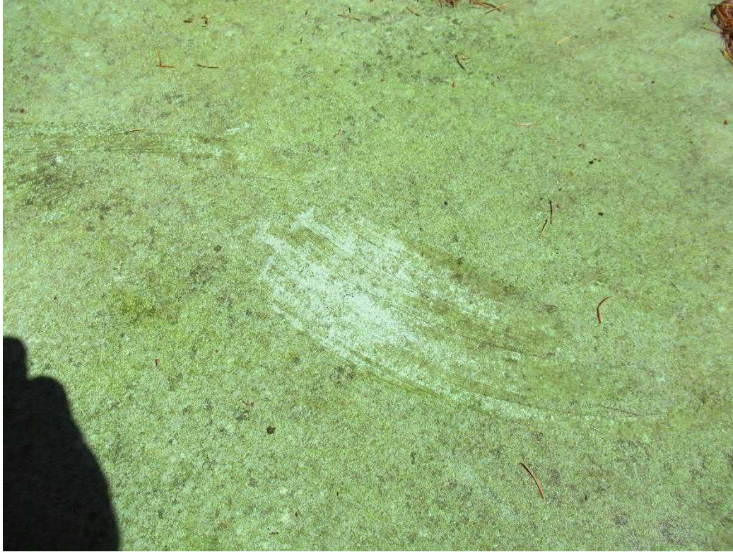
Photo 25: Closeup of the algae on the roof.
