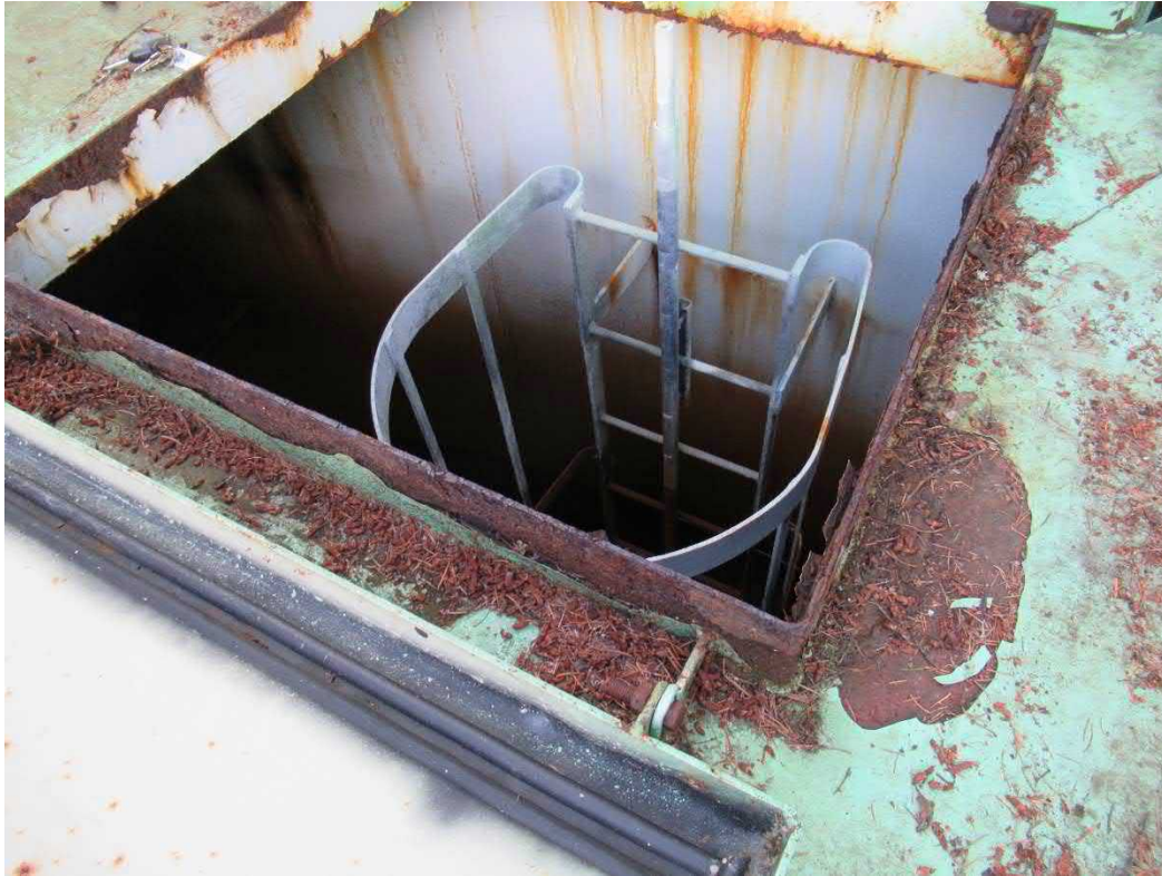
Photo 29: Inside of the access hatch.
