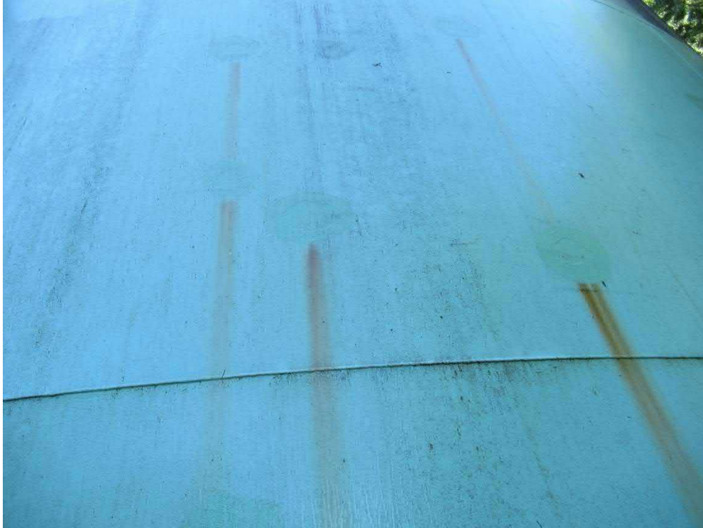
Photo 9: Rust stains from underneath coating patches.
