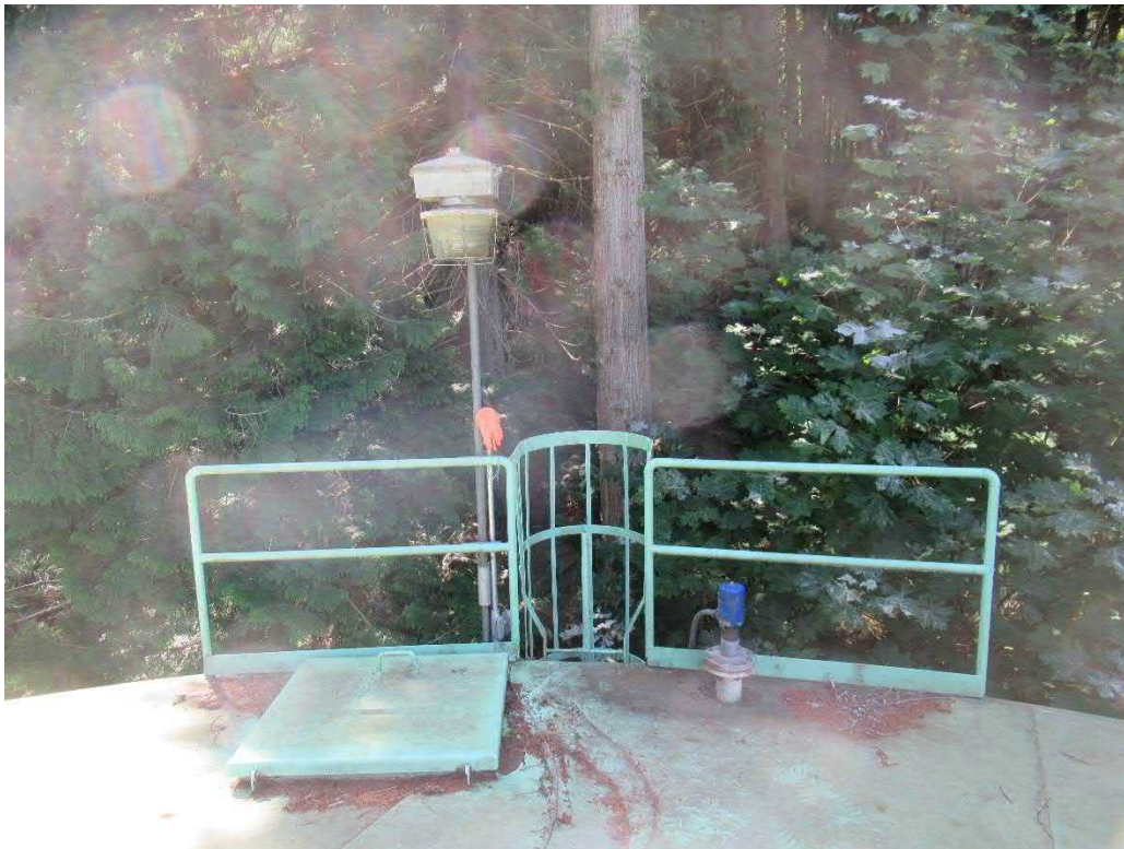
Photo 16: Ladder, railings, camera, and access hatch.
