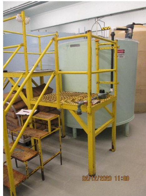
Soda Ash Storage Tank & Platform – Welded steel. Installed in 1992 and in good condition. Platform in fair condition while the mixer is in poor condition
