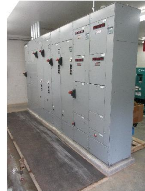
Seismic support – Example of MCCs with insufficient seismic support
