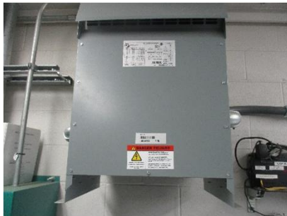
Seismic support – Example of wall mounted with insufficient seismic support
