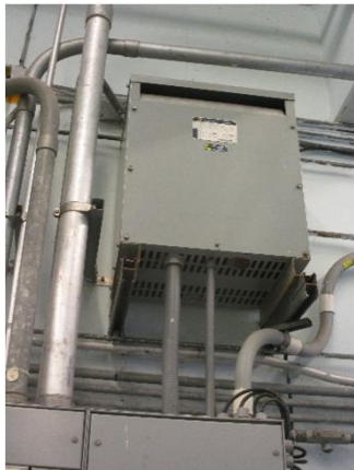
Seismic support – Example of equipment with insufficient seismic support
