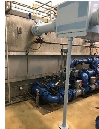
Seismic support – Example of piping with insufficient seismic support
