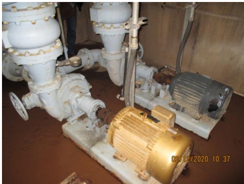
Raw Water Pumps – Raw Water Pump 2 is original (1970) and near the end of its recommended useful life.
