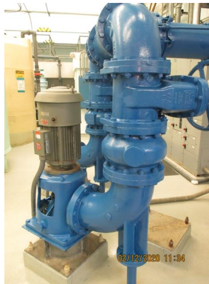
Transfer Pumps – Pumps are original (1990) and near the end of their recommended useful life.
