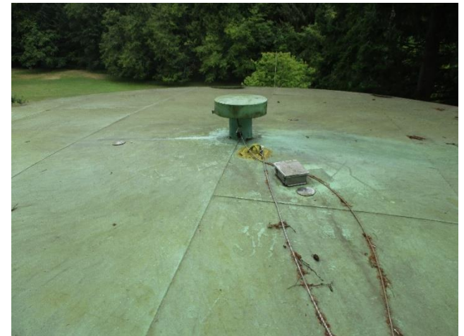
Algae – Roof exhibits lichen and algae growth, both of which may have damaged the coatings.
