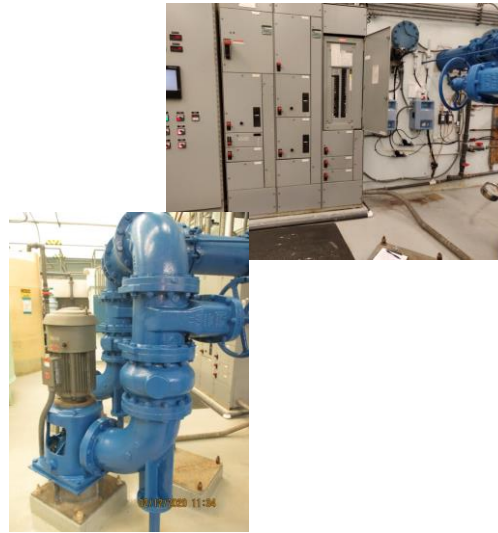
Transfer Pumps – Pumps are original (1992) and near the end of their recommended useful life.
