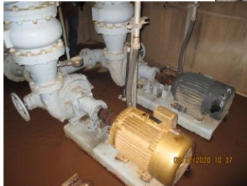
Raw Water Pumps – Raw Water Pump 2 is original (1972) and near the end of its recommended useful life.
