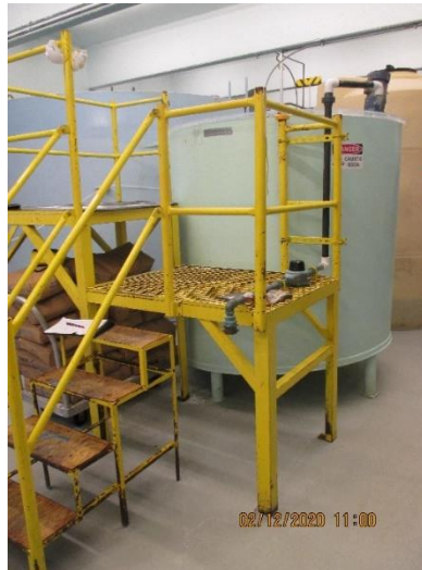
Soda Ash Storage Tank & Platform – Welded steel. Installed in 1992 and in good condition. Platform in fair condition while the mixer is in poor condition
