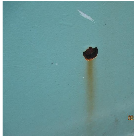
Corrosion – Tank has several corrosion spots, some of which have been repaired.
