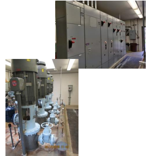
Finished Water Pumps – Pumps are original (1992) and near the end of their recommended useful life.
