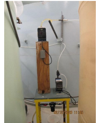
Metering Pumps – Lack of features requires daily manual calibration.
