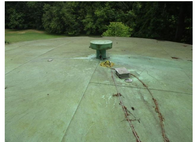
Algae – Roof exhibits lichen and algae growth, both of which may have damaged the coatings.
