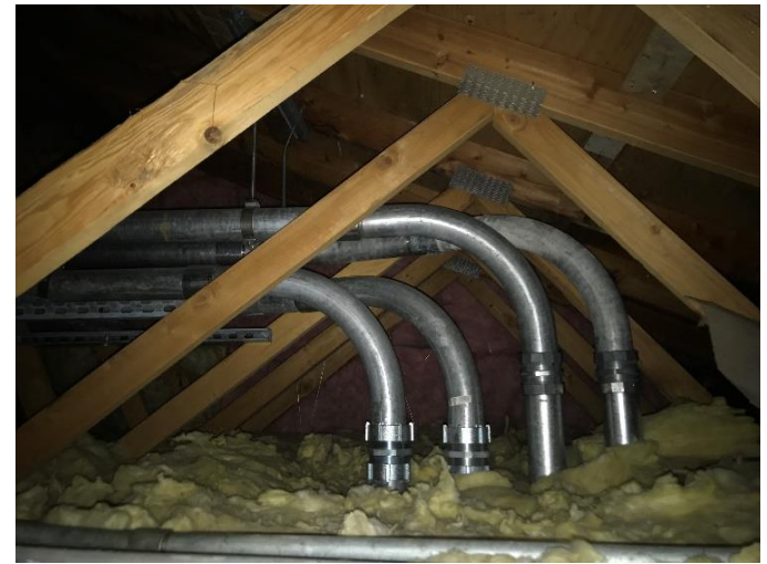
Seismic Support – Conduit within the FWP Building with insufficient seismic bracing.
