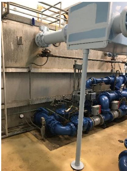
Seismic support – Example of piping with insufficient seismic support
