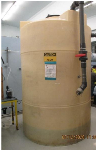
Alum Storage Tank – HPDE. Installed in 1992 and beyond its recommended useful life (15-17 years).
