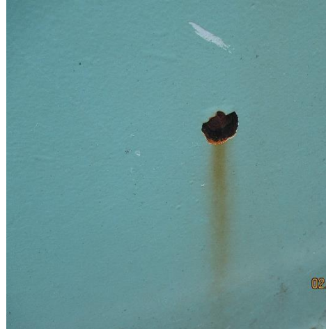
Corrosion – Tank has several corrosion spots, some of which have been repaired.
