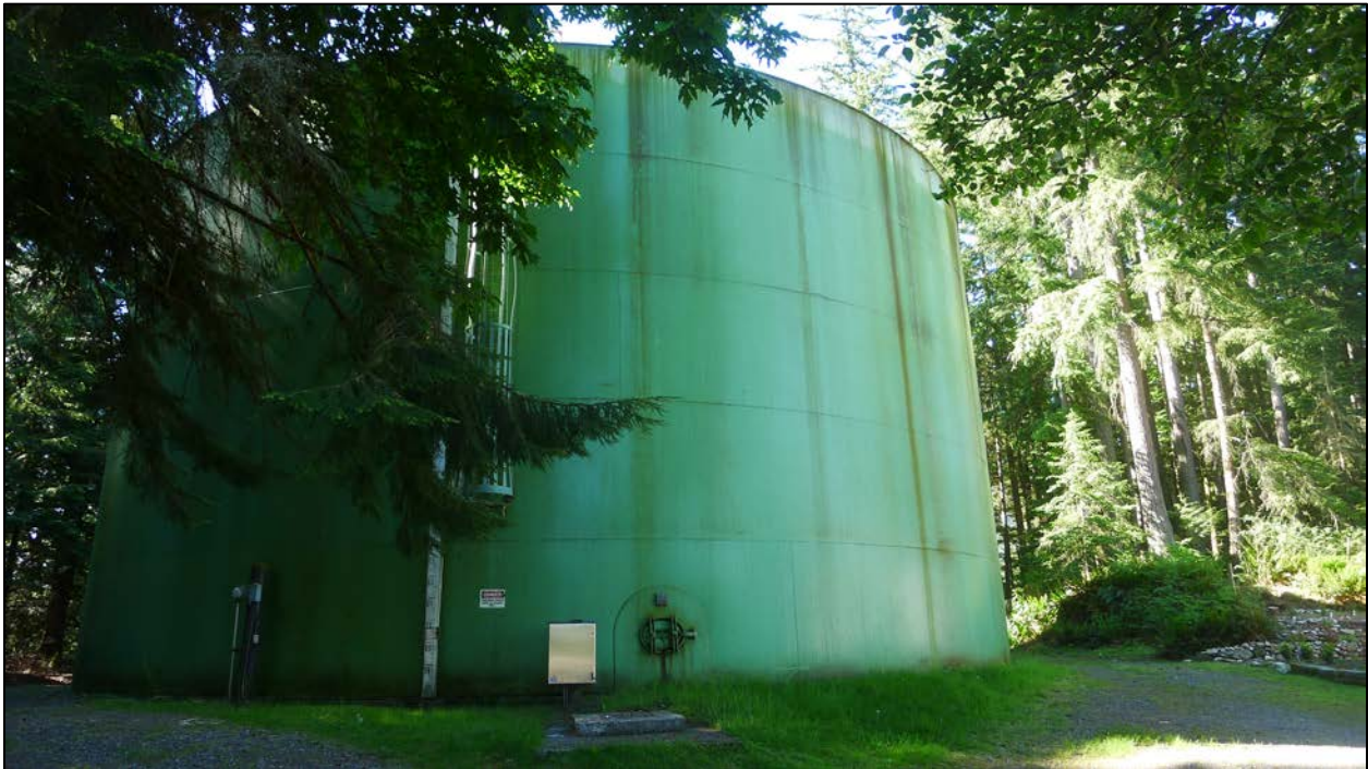
Figure 8. North side of existing reservoir showing level gauge, ladder, and access hatch. View to south.
