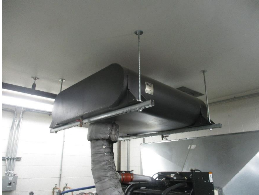
FIGURE B-1 Generator Exhaust
