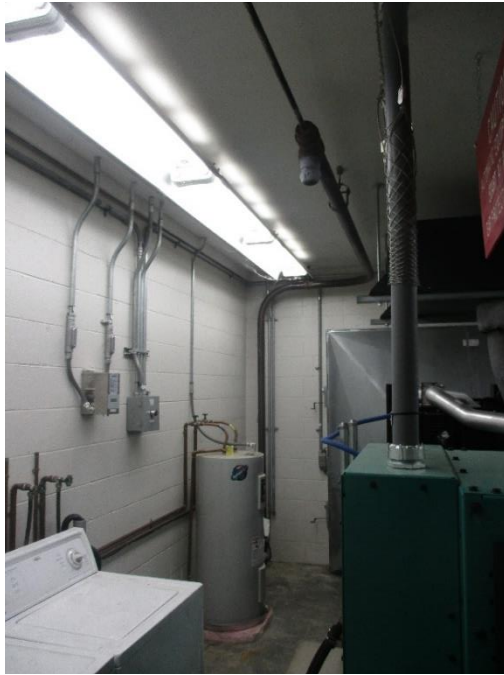
FIGURE B-7 Water Heater
