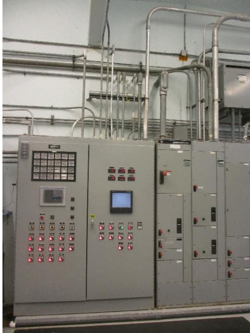
FIGURE A-5 Electrical Panels
