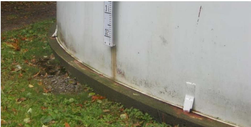
Figure 5 Geneva Reservoir at Shell to Foundation Interface
