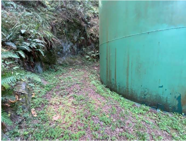
Mildew growth and ringwall below grade.
