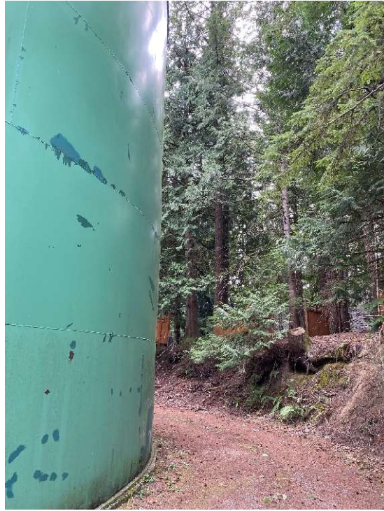
Delamination and repair areas.
