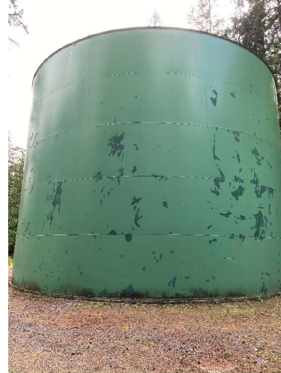
Delamination and repair areas.
