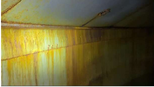
Mild corrosion and rust staining on the shell wall.
