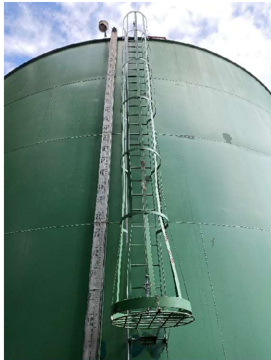
Ladder, cage, and level gauge.
