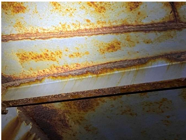
Rafter and roof plate corrosion.
