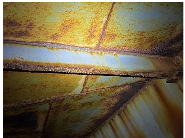
Severe corrosion of the upper and lower flanges.
