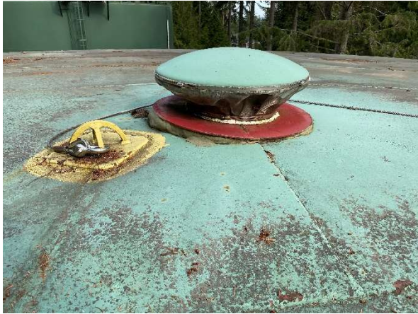
Roof vent and anchor.
