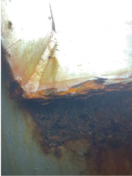
Moderate corrosion under the hatch riser.
