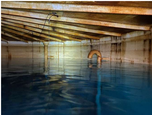
Inlet and Overflow
