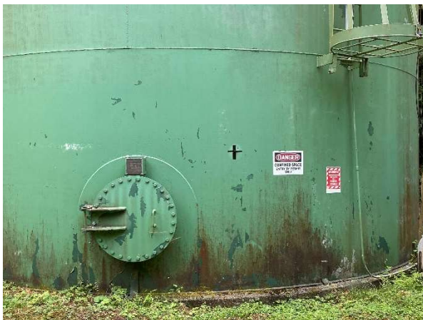
Access hatch and delamination areas.
