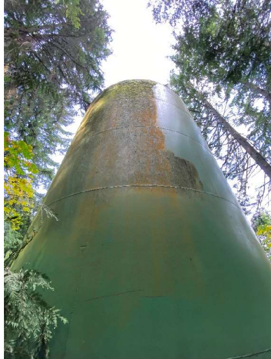
Moss growth on the shell wall.
