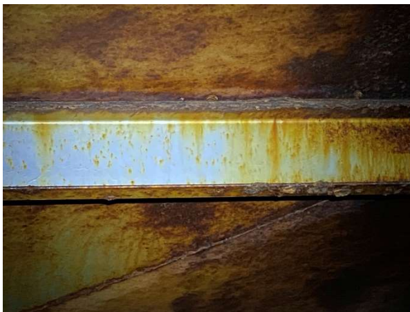
Severe corrosion of the upper flange.
