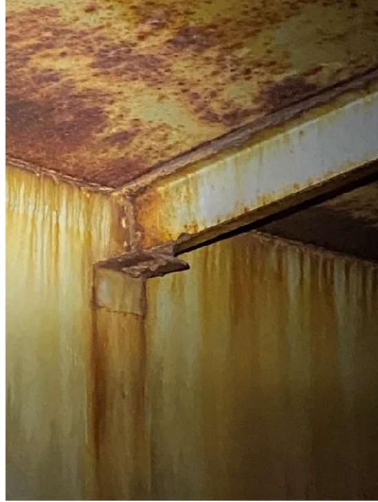
Bolts to the angle bracket have corroded away.
