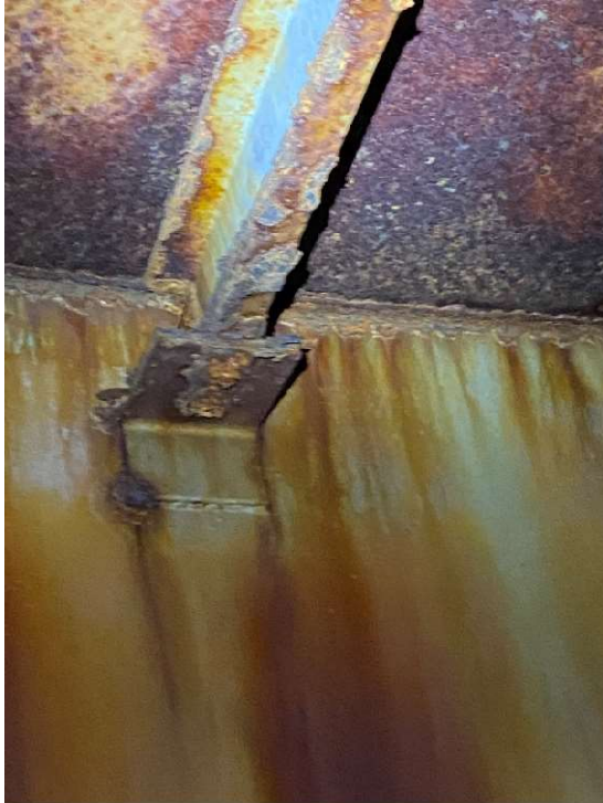
Corroded angle bracket, rim angle, and rafter.
