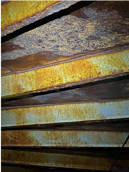
Corrosion on upper and lower flanges.
