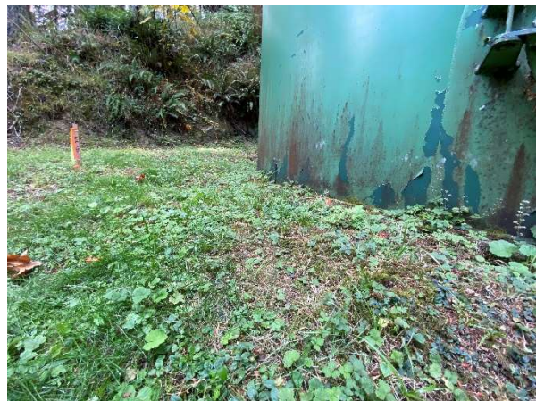
Shell wall delamination.
