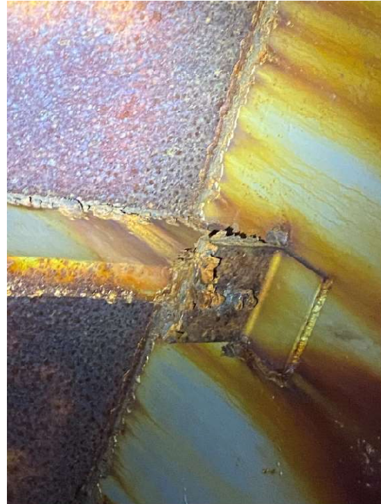
Corroded angle bracket, rim angle, and rafter.
