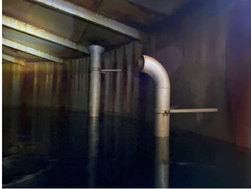
Staining on the wall in 2022.
