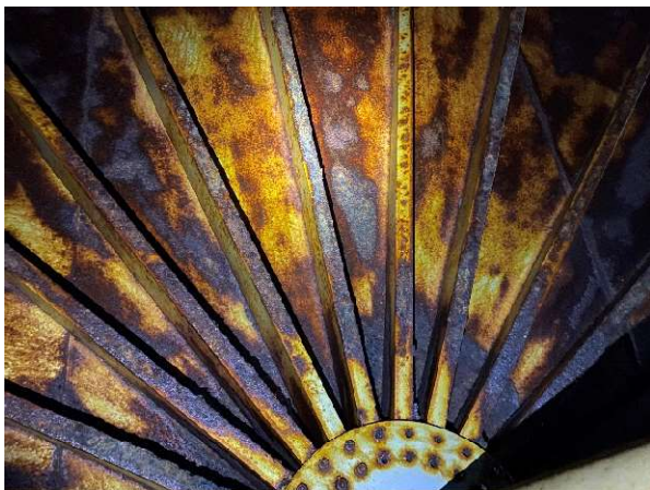
Rafter corrosion at the dollar plate.
