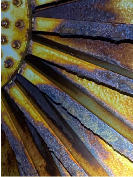
Severe corrosion on upper and lower flanges.
