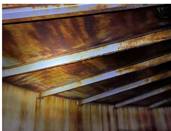
Rafter and roof plate corrosion.
