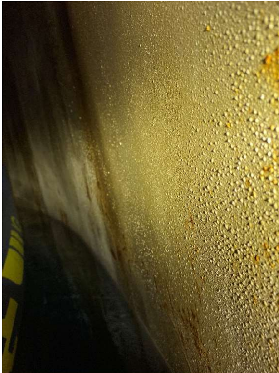
Coatings on the shell wall heavily blistered.
