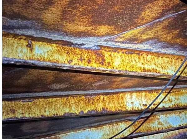
Rafter and roof plate corrosion.
