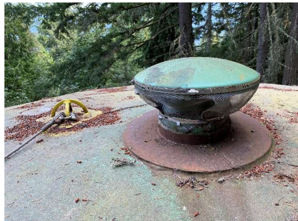
Roof vent and anchor.
