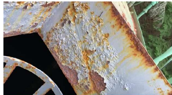
Moderate corrosion on the access hatch riser.
