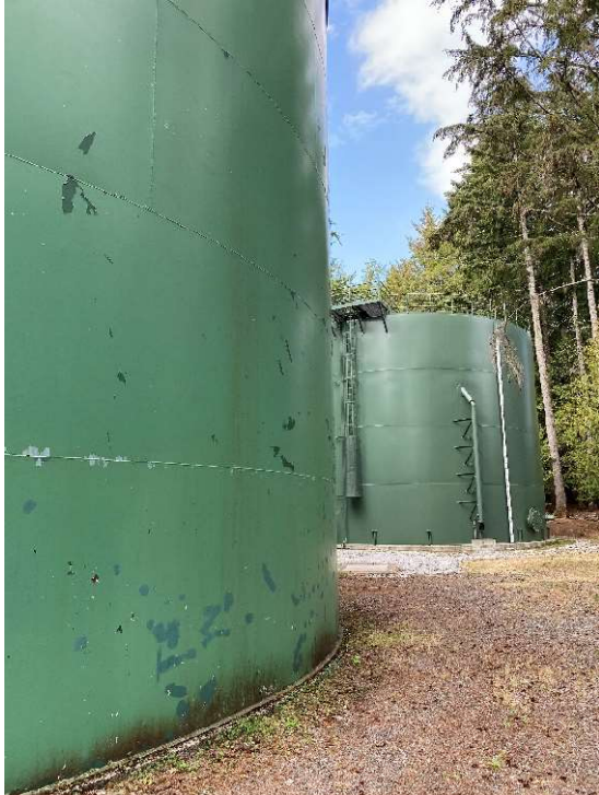
Delamination and repair areas.
