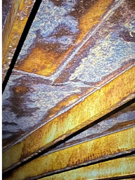
Severe corrosion of the roof plates and rafters.
