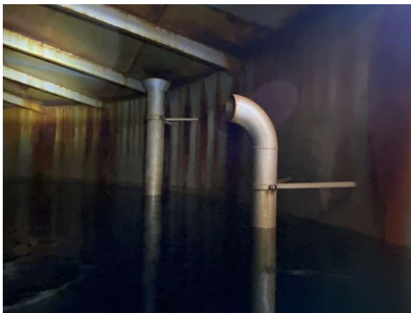
Inlet and Overflow
