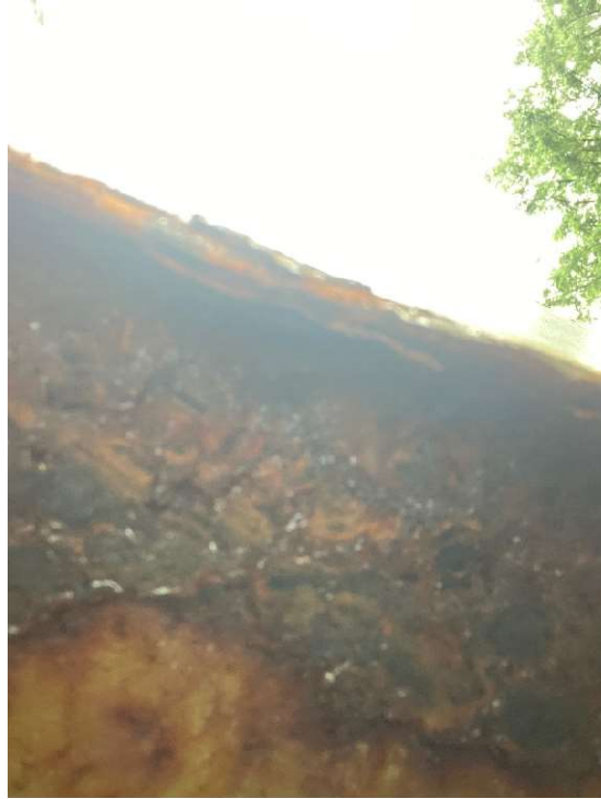
Moderate corrosion under the hatch riser.
