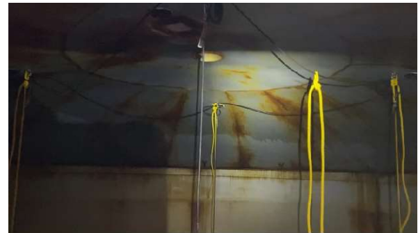
General rusting of the roof plates.
