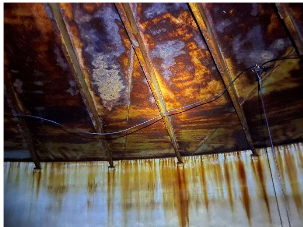
Rafter and roof plate corrosion.
