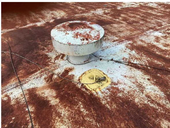
Roof vent and anchor.
