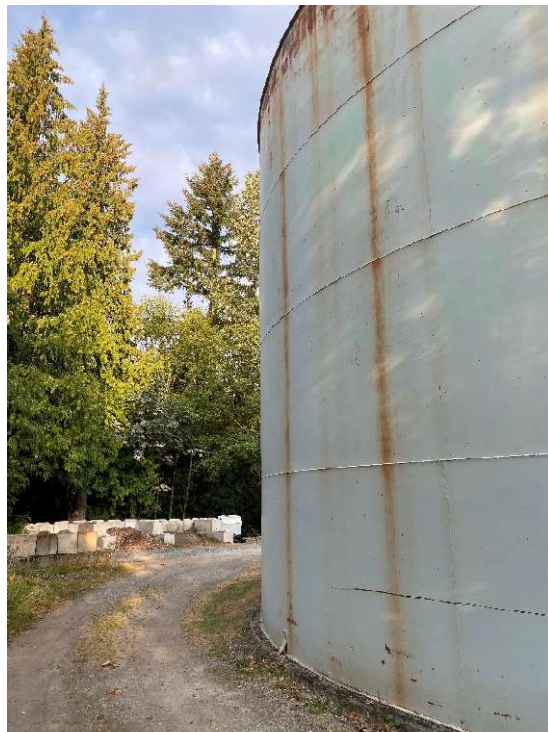
Corrosion beginning at the top of the shell wall.
