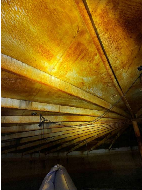
Mild corrosion of the roof plates and rafters.
