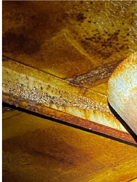
Moderate corrosion on the rafter and roof plate.
