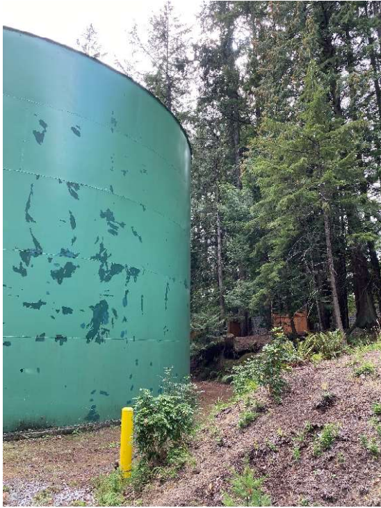
Delamination and repair areas.
